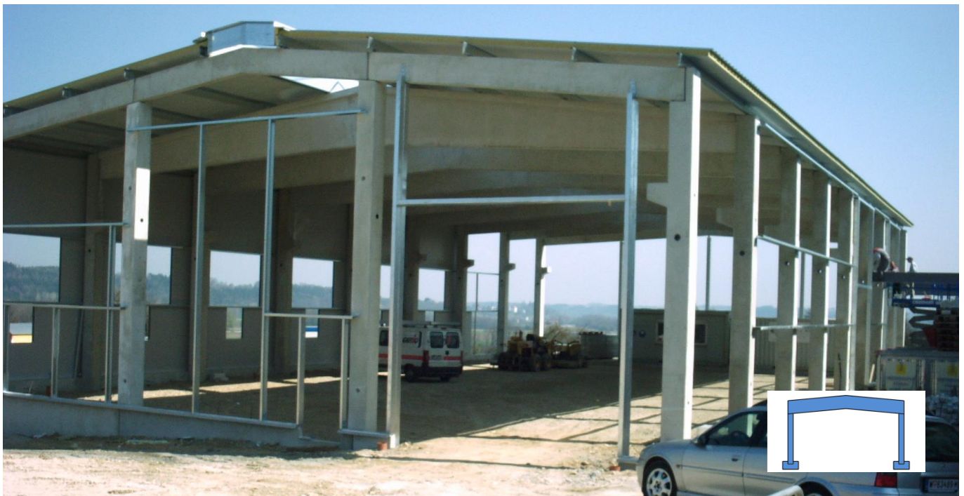
Figure 6: Single storey building with a precast RC frame, symbol for RC frame
